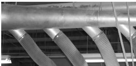
Multi-Tap Manifold (4 taps) for a sander used in a custom cabinet facility.
