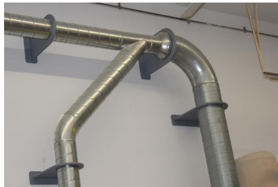
Connection to Dust Collector
