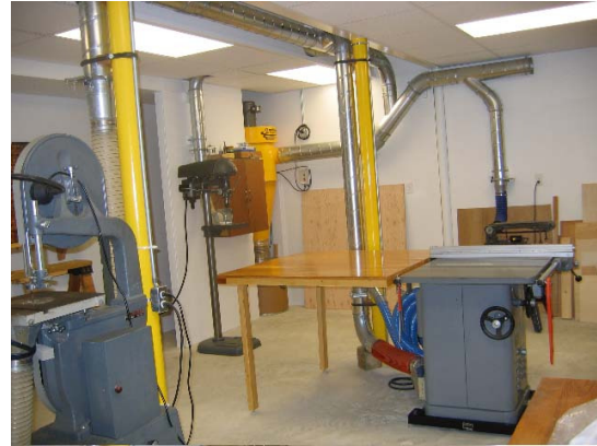
Hobby Shop Ductwork
