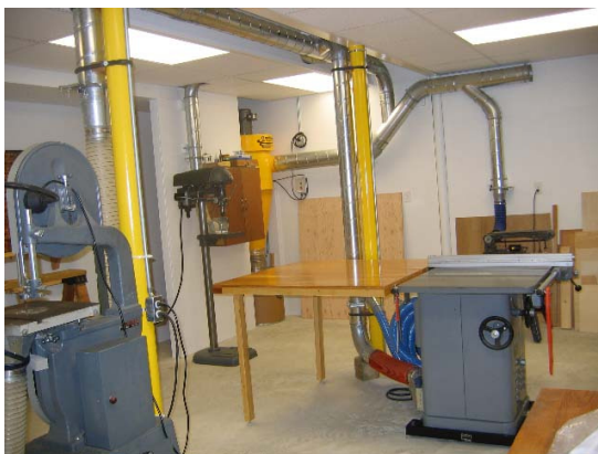
Hobby Shop Ductwork
