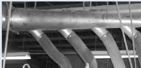
Multi-Tap Manifold (4 taps) for a sander used in a custom kitchen cabinet facility.
